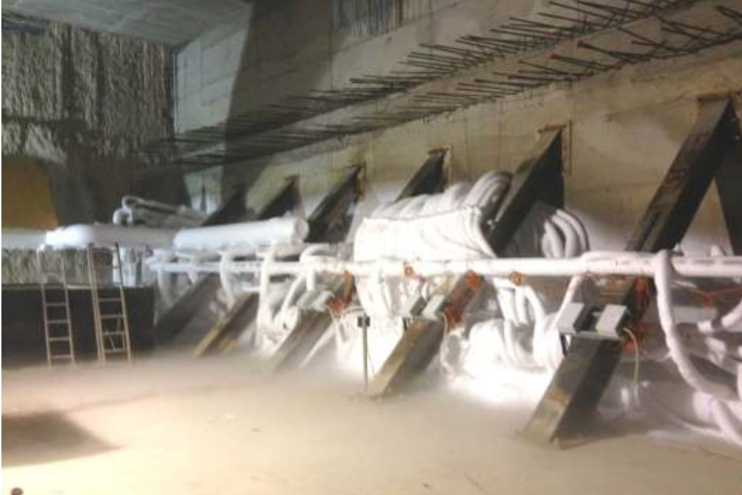
Liquid nitrogen installations - West Shaft
